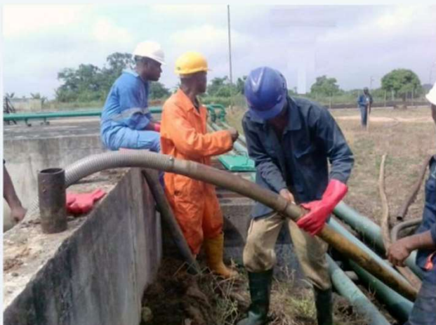
Extension of hoses to safer pit to facilitate Crude oil recycling from sludge
