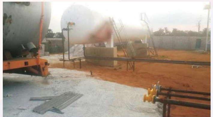
Abegas, LPG Plant, Port-Harcourt
