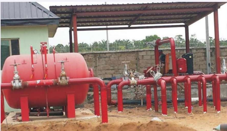
Fire Safety Installation
