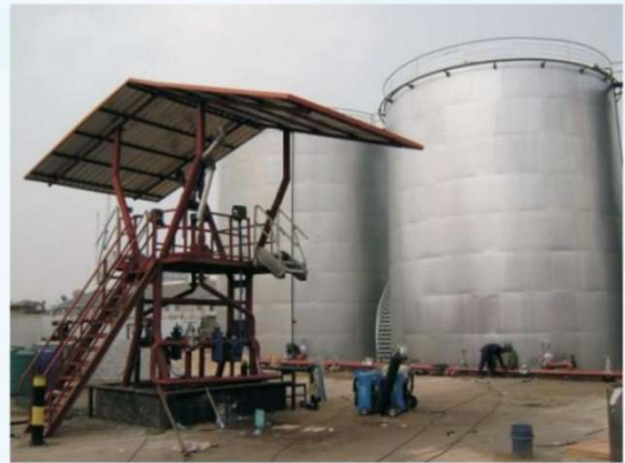
Mettle Tanks & Gantry
