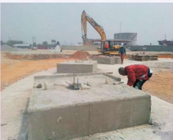
LPG Cylindrical Tank support base.
