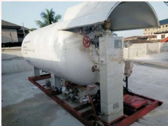
Skid Mounted LPG Tank
