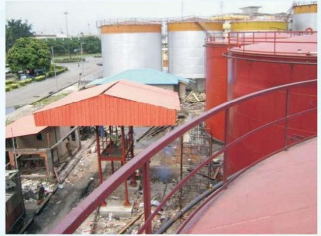
Completed Petroleum Storage Tanks
