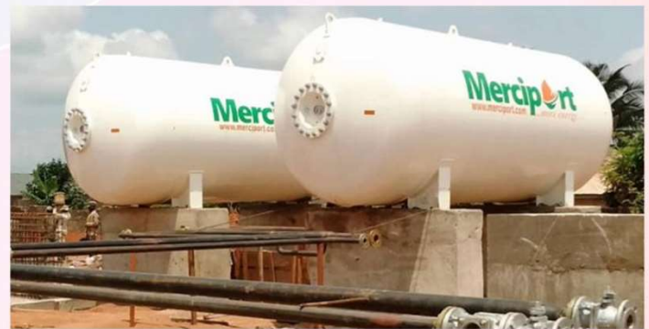
MerciPort LPG Plant Tanks
