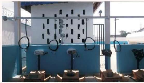
Matrix LPG Plant, Filling Platform.
