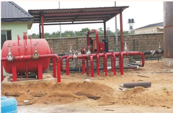
Gonzaga Fire fighting/Safety Installation
