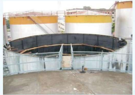
SPOG Petroleum Products Storage Tanks
