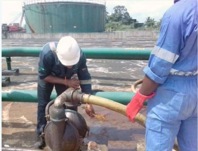
Tightening of hoses to diaphragm pump for de-sludging operations of the crude oil tank
