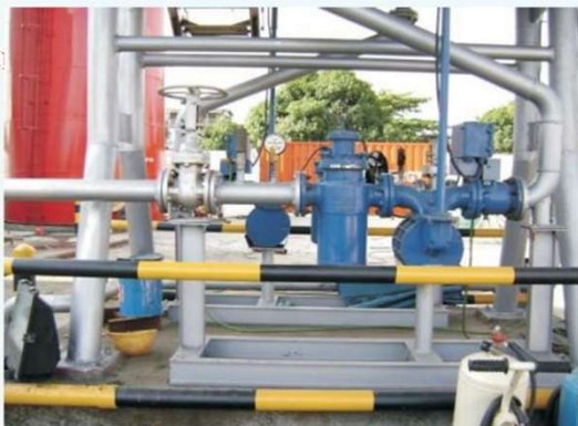
Gonzaga Petroleum products piping Network
