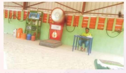
Unity Gas, Filling platform, Port-Harcourt
