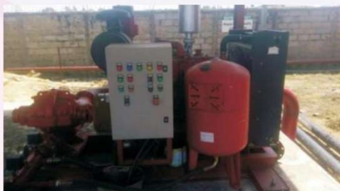
Diesel Fire Pump
