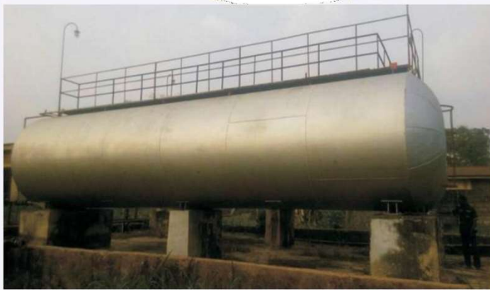
Citigas, LPG tank Installation, Ekpoma
